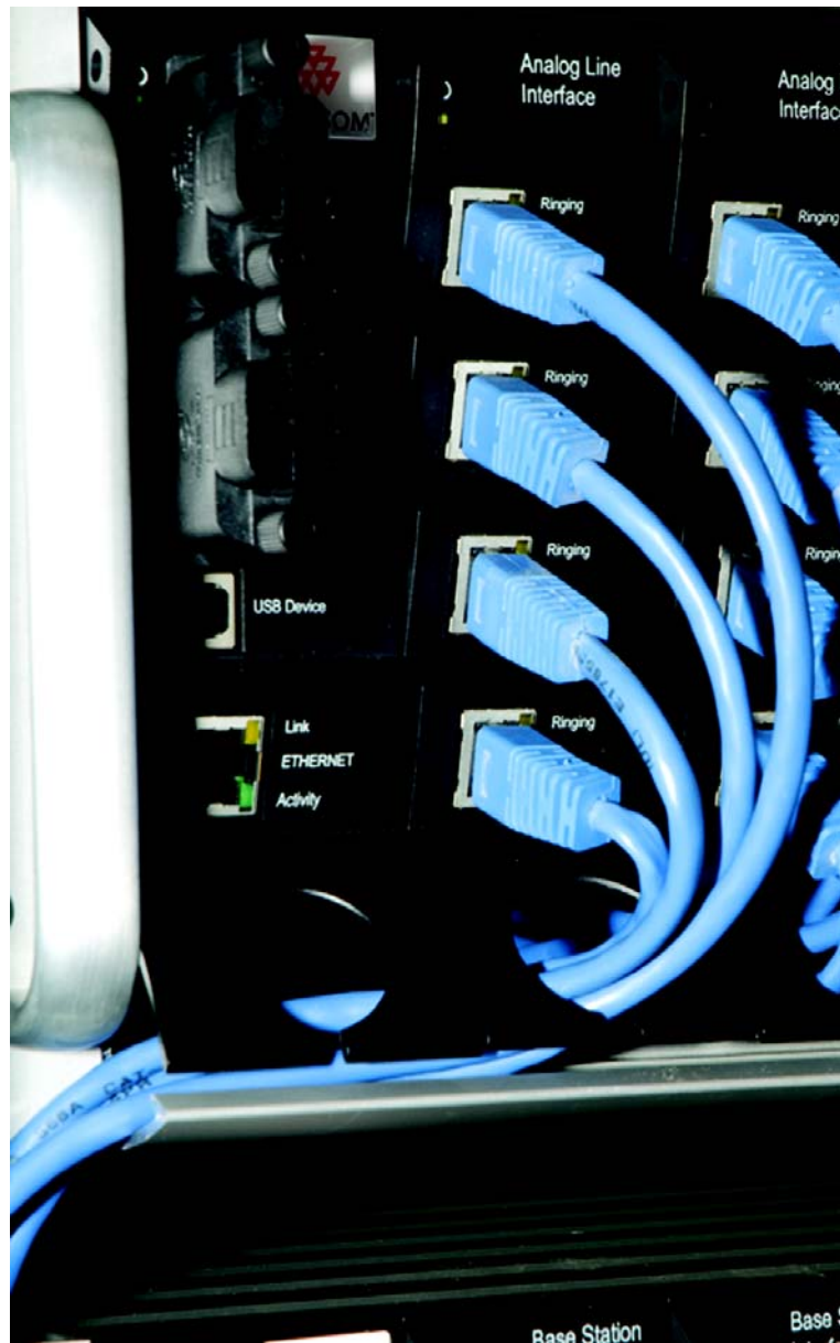
Figure 12 Harnessing cables to the side and out.
